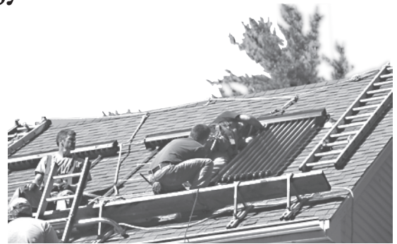
Volunteers and the homeowner install one of the 50 Apricus tubes, the last step in the process.
